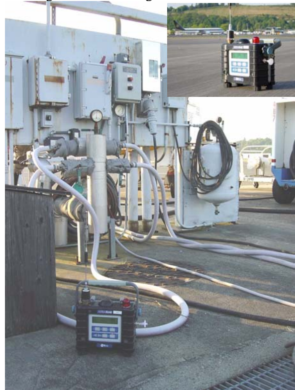
Figure 6. AreaRAE monitoring Boeing Airfield fuel pumping station during TOPOFF II.
