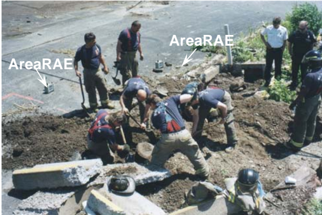
Figure 3. Perimeter monitoring during repair of leaking gas pipe (propane is explosive, but not highly toxic).
